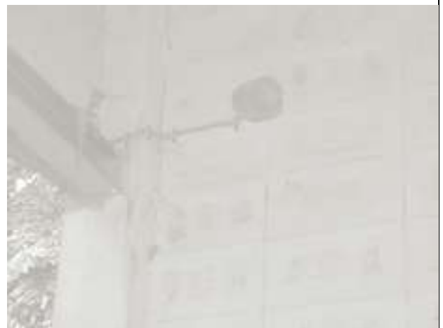
Fire alarm in workshop
