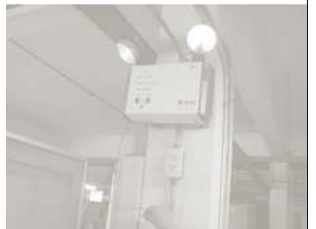
Emergency lighting in workshop
